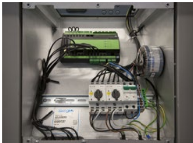
All electrical and control equipment is collected inside a special enclosure in the centred section of the air handling unit.
